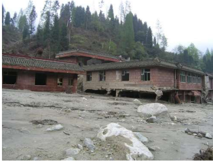
Fig. 19. Buildings in Yinchanggou Gully destroyed by debris flow during post-seismic rainfall.
